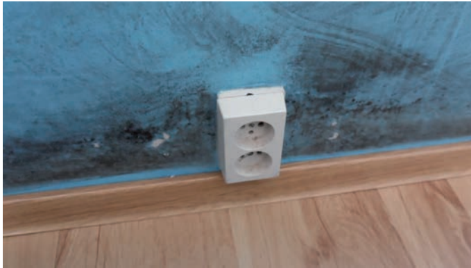
II. 2. Moulds around an electrical socket and skirting board on the ground floor (the author).
