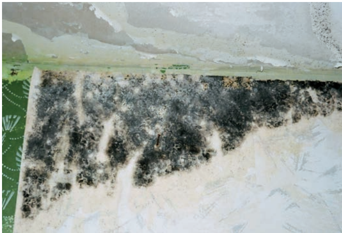
II. 3. Moulds on a wall of a room under the ceiling - after "flooding" (the author).
