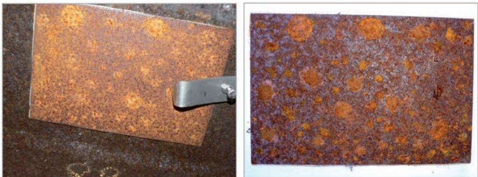
Figure 6: Samples of top flange bottom surfaces P4 after 1 year (left) and 3 years (right)
