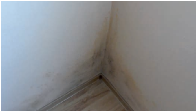
Il. 5. Dampness and mould in a corner of a room on the ground floor (the author).
