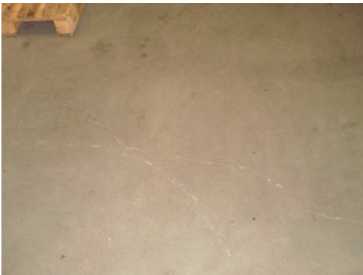
Figure. 11 Cracks on the floor
