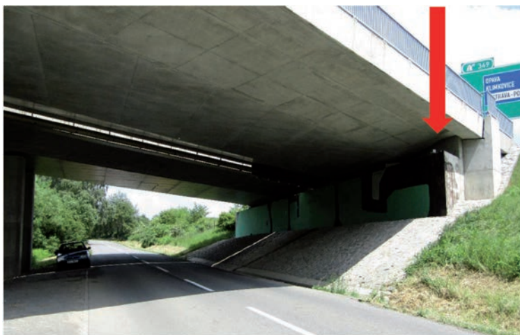
Figure 9: The concrete bridge construction across the street Vřesinská (the bridge is located below the D1)
