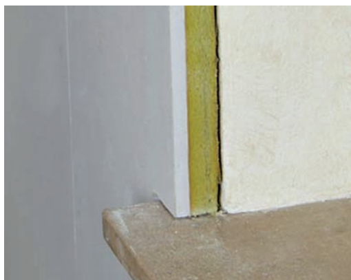
II.2. Aerial as insulation from the inside (Materials by Deutsche Rockwool Mineralwool. www.Aerowolle.de )
