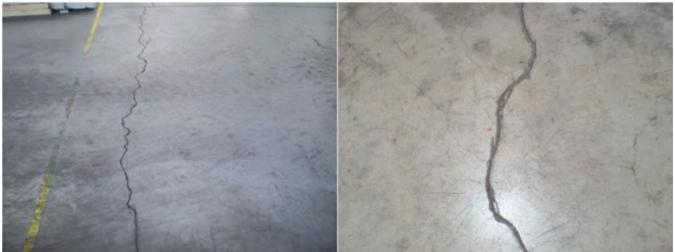
Figure 5 Cracks near the entrance (V1 and V2)
