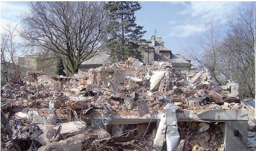
II.1. Demolition of the building – the diversity of waste material, photo Mohamed Ahmad, 16.06.2016
