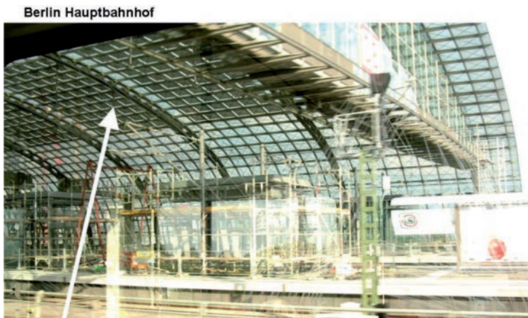
II.3. Photovoltaic components installed on the glass roof of the central railway station in Berlin. (photo Anna M. Włodarczyk, 2014)
