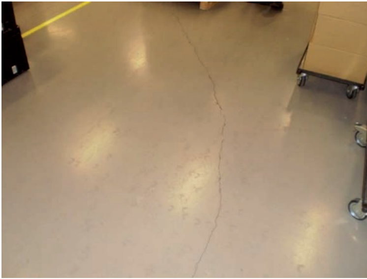
Figure. 10 Cracks on the floor
